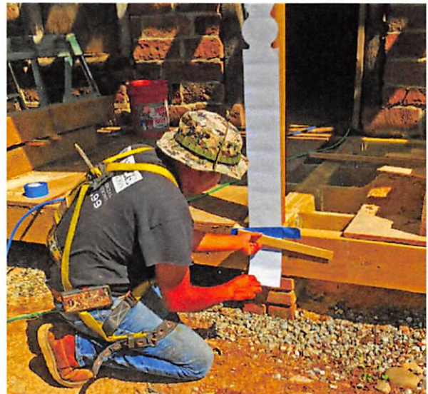
Many projects on historic buildings include a range of actions from maintenance through replacement.
