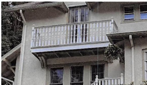
A necessary and highly visible balcony support becomes a visual asset through good exterior detailing.
