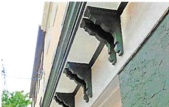
Brackets provide a graceful transition at eaves and overhangs. Wood details are traditional; plastics and composites need close attention to their greater expansion and contraction properties to avoid problems.
