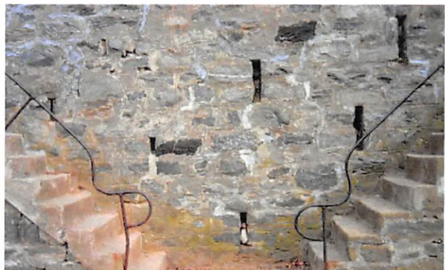
Age-old retaining wall and steps. Random weep holes deal with underground water pressure.
