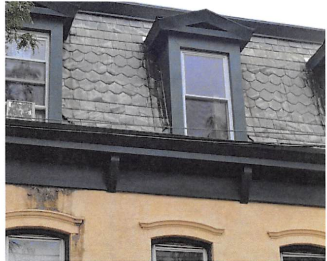
Luckily, many important buildings retain original materials that lend enormous character and texture to the streetscape. When maintained, natural materials like the slate shown here last a century or more.
